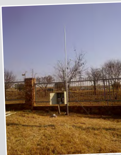
Wireless Repeater Station
