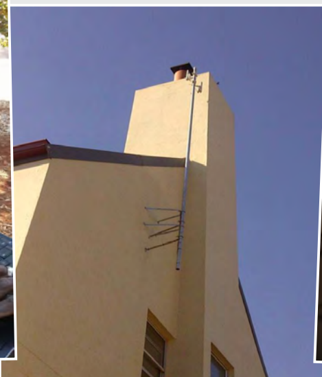
Wireless Antenna at Control Room
