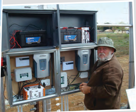
JVA security installation, Africa
